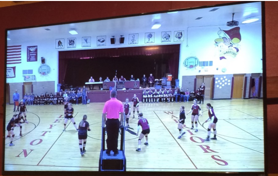
TV and Video Equipment in Multi-Purpose Room
